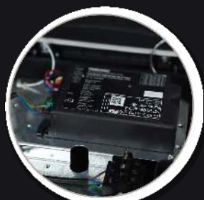
Driver compartment — removable wiring plate
